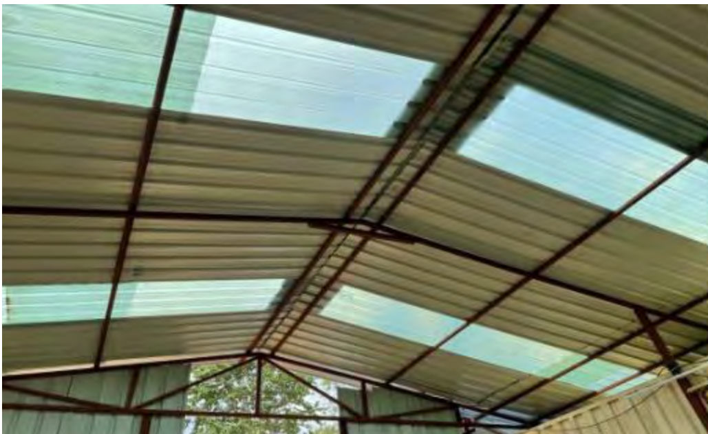
Using transparent sheet in store and other sheds to reduce electricity consumption.
